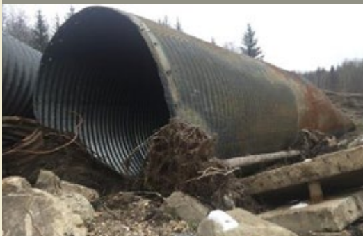
Exhibit 6: One of the culverts damaged in the June 2016 storm in the Peace region of B.C.
